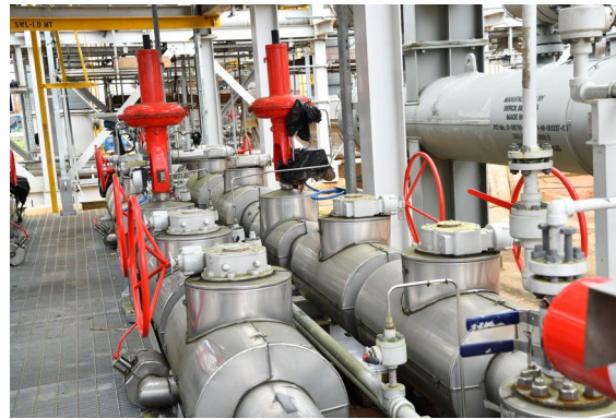
JOULE THOMPSON (JT) VALVES SKID - TRAIN 2
