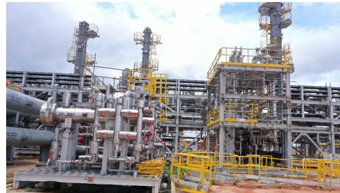
LOW TEMPERATURE SEPARATOR, COALESCER & FUEL GAS SKID
