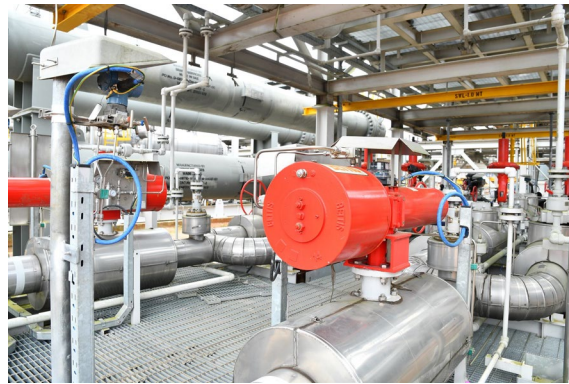
JOULE THOMPSON (JT) VALVES SKID - TRAIN 1
